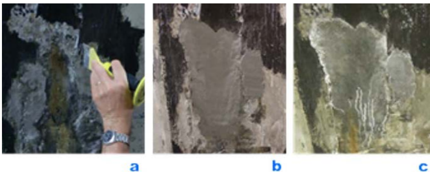
Figure 3. Self-healing mortar applied in practice: a) Surface preparations, b) Application, c) Visible limestone formation (white lines) on the surface of the set repair mortar [7]
