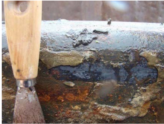
Figure 5. Crusts of mineral deposits formed by microbial communities on the surface of sheet pilings. Image courtesy of Michael Asanajef, Delft University of Technology
