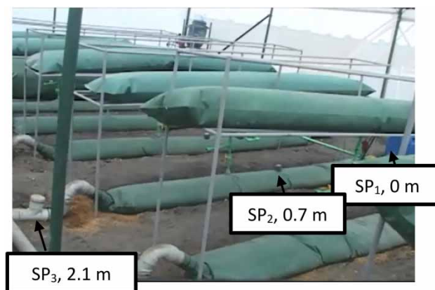
Figure 1 | Plug flow digester layout; digesters on the floor, biogas collection bags directly above; sampling points at different length of the digester are indicated as SP 1 , SP 2 and SP 3 , respectively.
