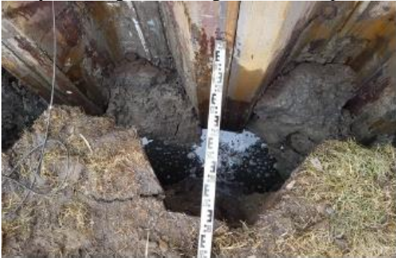
Figure 16. Gapping behind sheet pile wall AZ26
