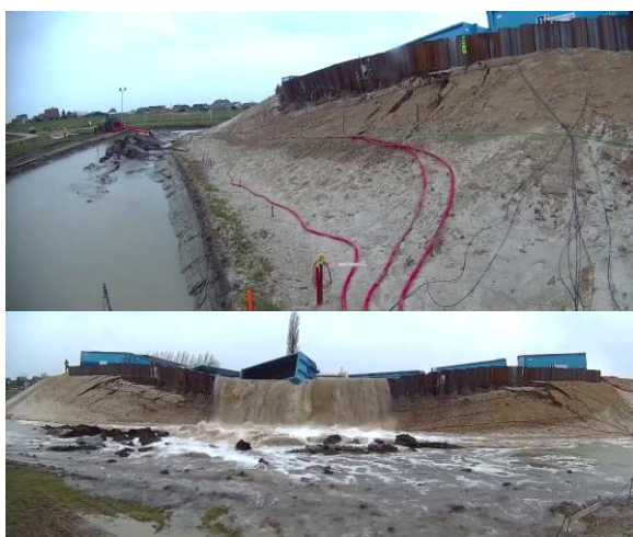
Figure 12 Photo's of sheet pile dike during failure, just before (a) and during (b) flooding.
