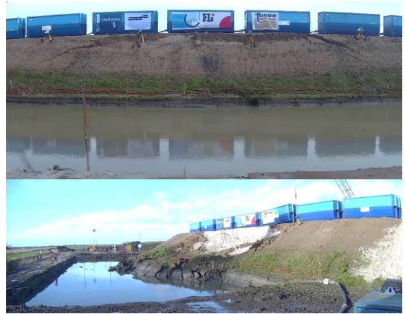
Figure 9 Photo's of ground during failure (a) and after failure (b).
