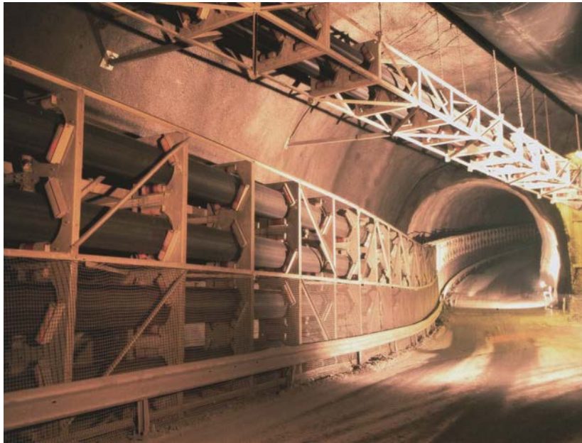
Figure 1.4: Pipe conveyors transporting bulk solids through a narrow tunnel passage during the construction of Lötschberg base tunnel in Switzerland (Image courtesy FLSmidth Wadgassen GmbH).
