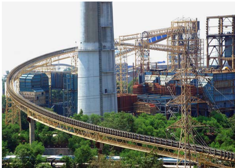
Figure 1.1: Double pipe conveyor system operating in Tata Power Plant, Mumbai, India (Image courtesy FLSmidth Wadgassen GmbH).
