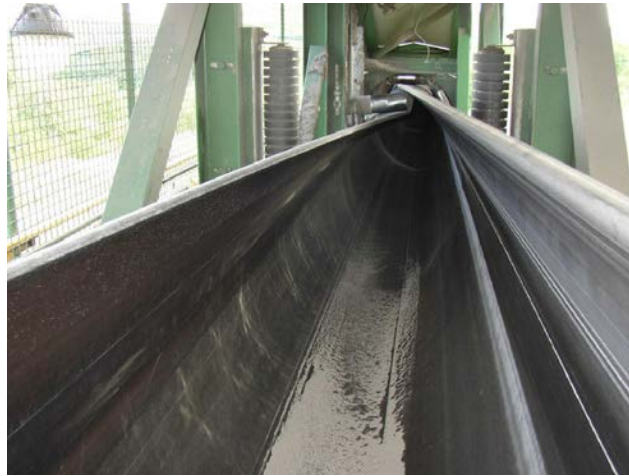
Figure 2.2: Folding belt from flat shape into a pipe shape (Image courtesy of Specialty Welding & Fabricating of New York, Inc.)
