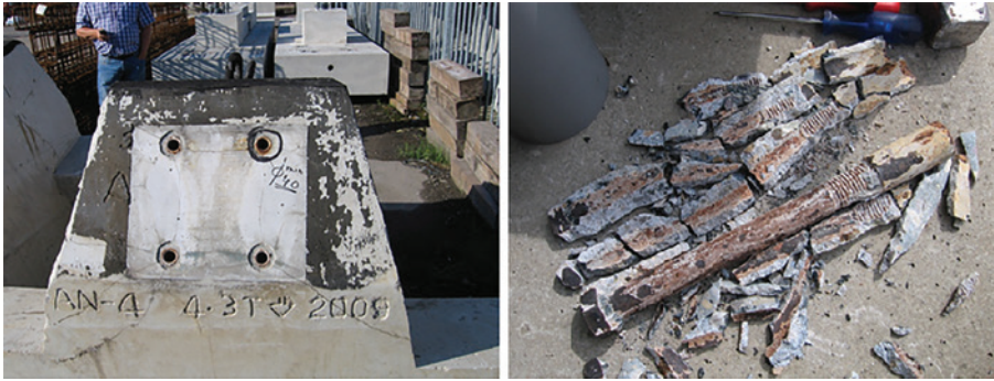
Figure 9: Damaged block due to the corrosion of anchor induced by stray current.
