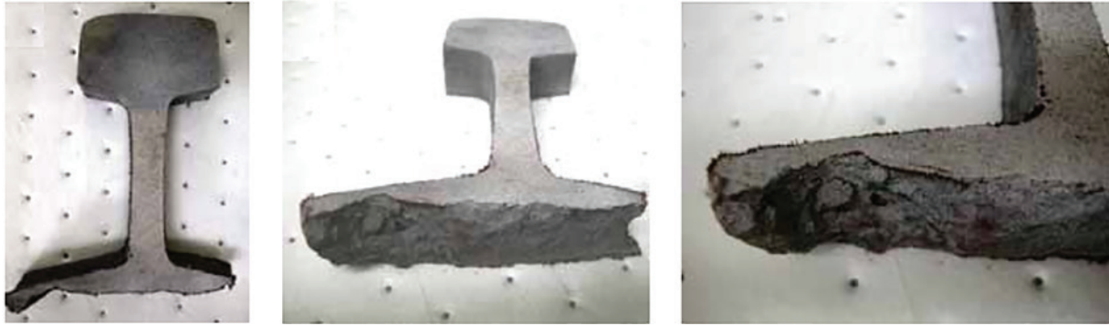
Figure 6: Different views of a section of 100 lb rail showing severe corrosion at the base of the rail (Francisco & Gabriel, 2007). Reproduced with permission from the National Academies Press.
