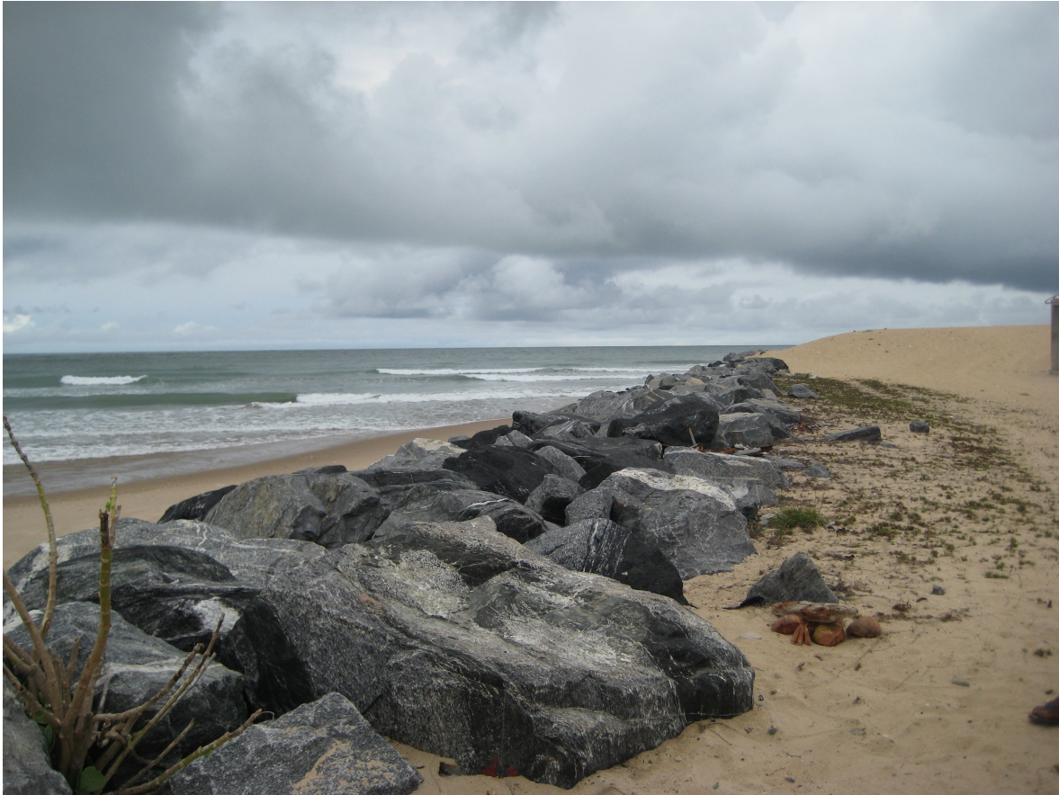
Figure 2-5: The Ada sea defence project, at Kewunor, looking south. Visible is the last groyne west of the Volta river mouth (to the left) and the beach barrier to the right. The spit used to extend across the river mouth, but has largely been eroded.
