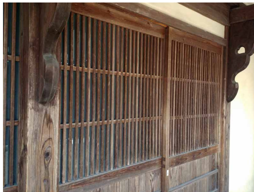
FIG. 3 Koshi placement close to the exterior window surface in a house, in Uchiko, Ehime
