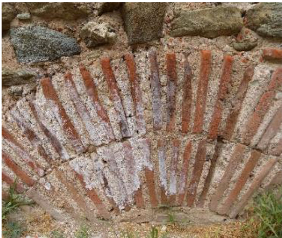
Fig. 31 Efflorescence near to the ground level
