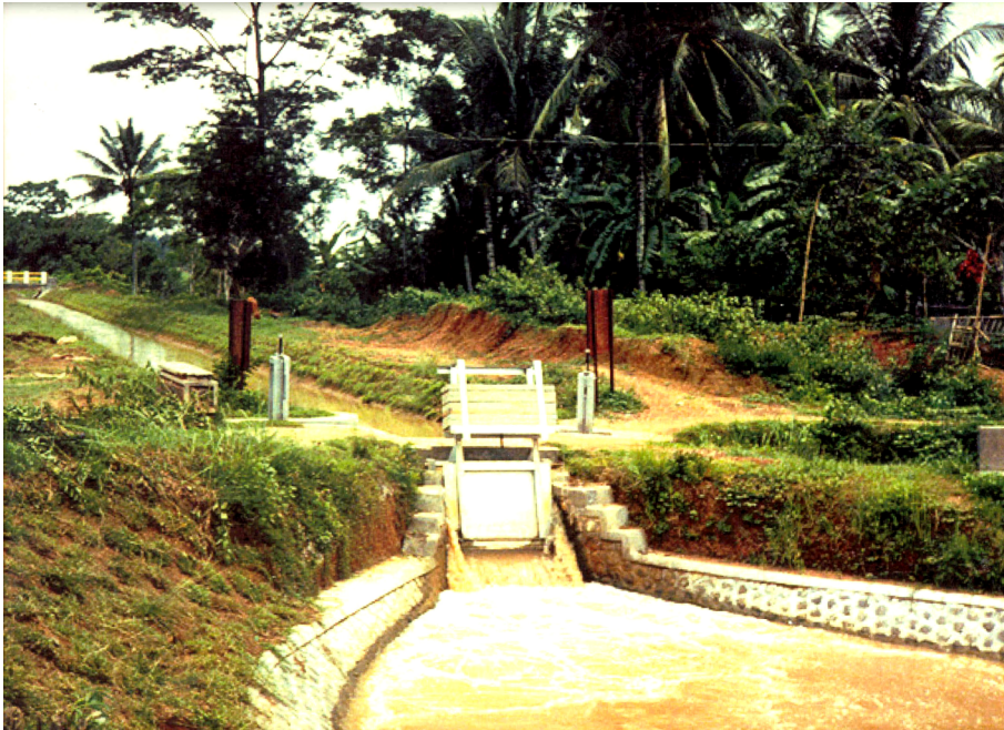
Figure 7.7 Begemann gate in the Punggur Utara system
