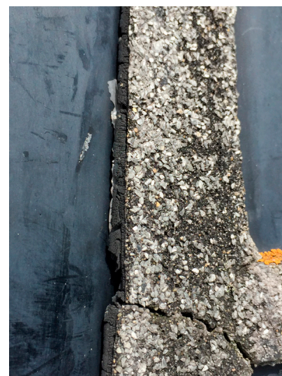
Figure 5. Exterior view of the glass-mortar interface at one dalle de verre slab, with a large adjacent mortar crack. Courtesy of Norman Tennent
