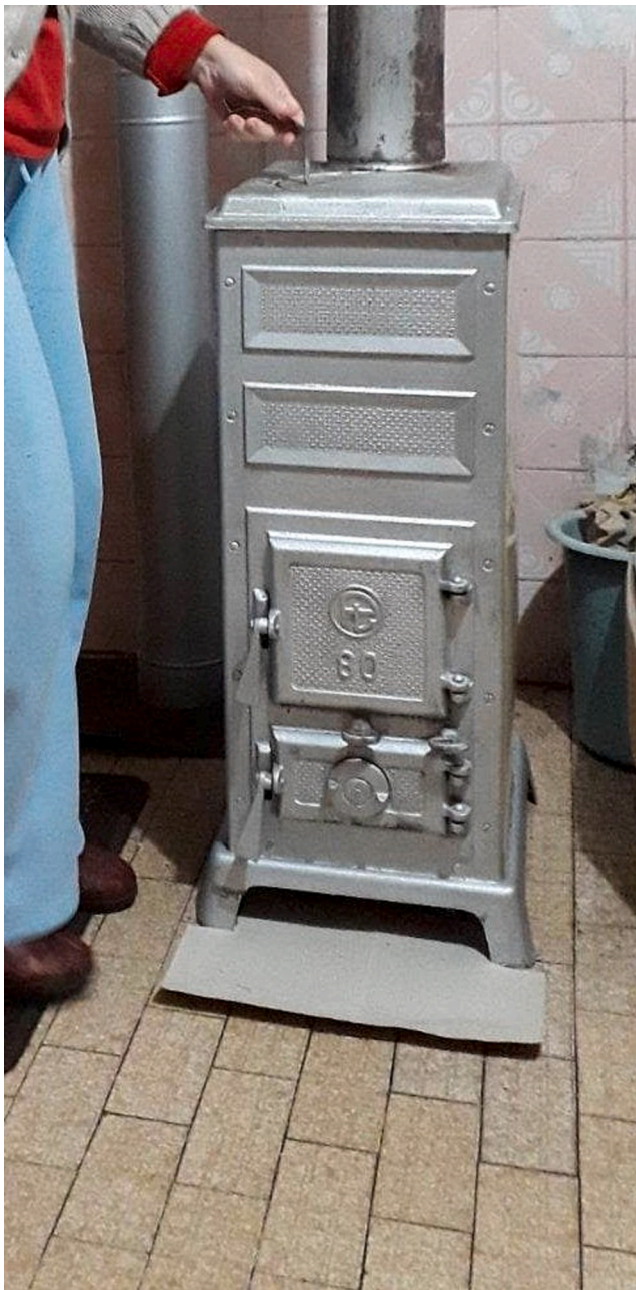
Fig. 5. Old-fashioned fuelwood stove in North Macedonia.
