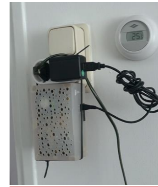
Figure 1: The monitoring boxes installed in the dwellings, developed by industrial partner OfficeVitae.
