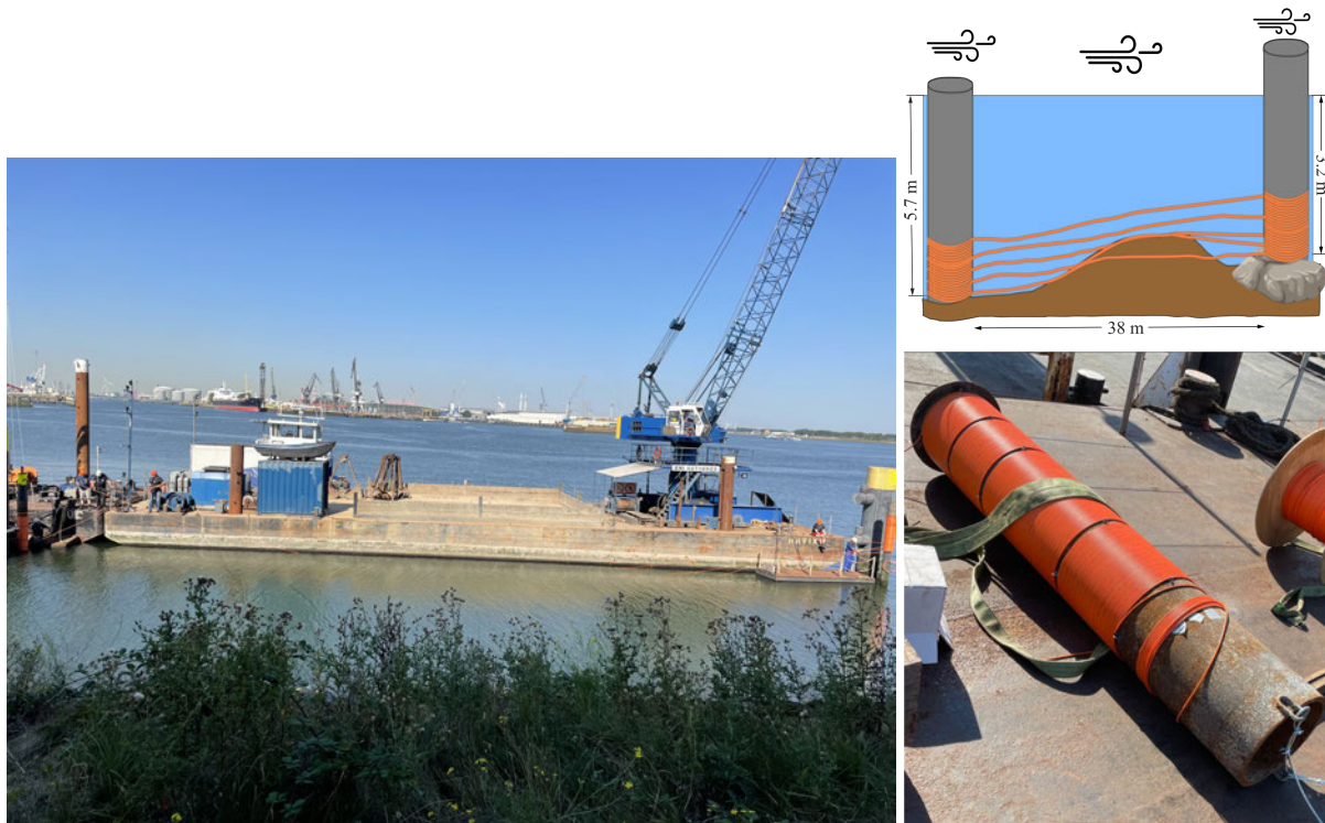
Figure 1 Left: two mantels with the direct burial single mode fibre being lowered onto the steel poles. Top and bottom right: sketch of the setup and a picture of a mantel with the fibre.
