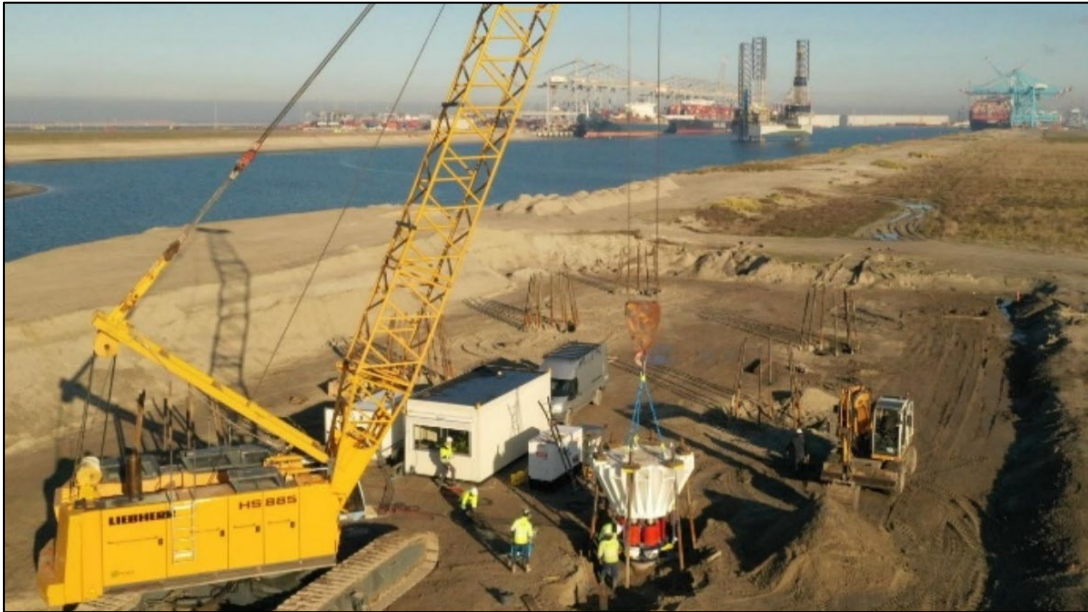
Figure 1: Lifting the load test frame into place at the Amaliahaven test site
