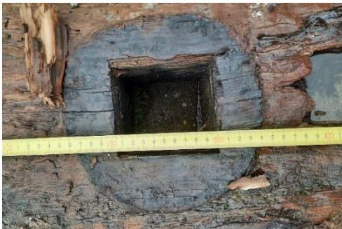
Figure 6.4, Headstock extracted from collapsed Grimburgwal with pin hole and pile imprint visible (Korff et al., 2021).
