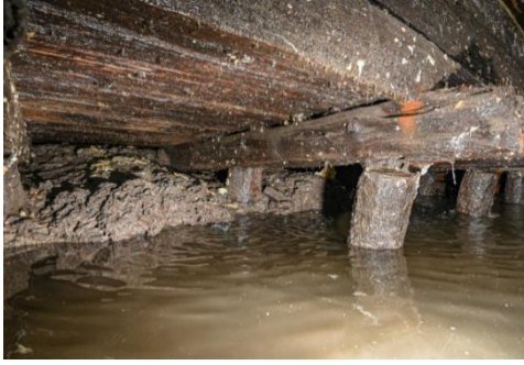
Figure 5.9, Photograph of pile-headstock connections below a historic quay wall in Amsterdam (Maarschalkerwaard, 2022).
