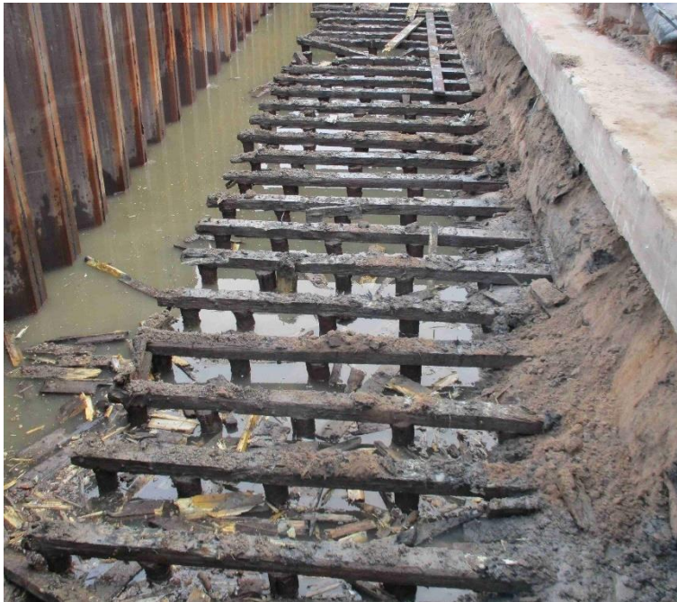
Figure 4.2, Excavated historical quay wall, 'Maaskade' in Rotterdam. Left of the pile foundation, the water is situated and right the hinterland used to be present. Photograph: Julianus, Eric. "Exposed timber pile foundation of the Maaskade". 2019. Havenbedrijf Rotterdam.
