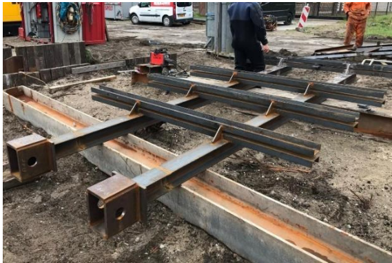
Figure 4.25, Steel frame to be installed underwater and connected with tension slings to the 3x4 pile matrix.
