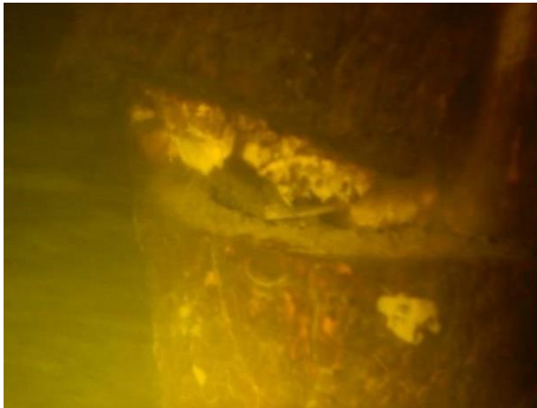
Figure 6.8, Diver photo of pile breakage (Baars-Cipro, 2021).
