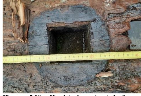
Figure 5.10, Headstock extracted from collapsed Grimburgwal with pin hole and pile imprint visible (Korff et al., 2021).
