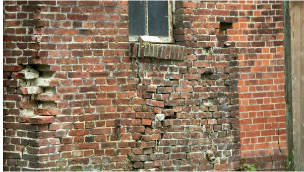
Figure 1.2: A house destroyed due to surface subsidence in Groningen. This figure is retrieved from [19].
