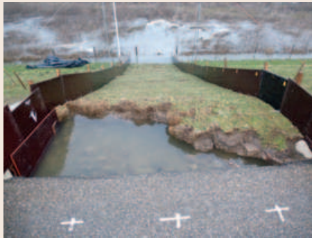
Figures 1 and 2 (below). Final scoured grass cover of a dike with a road after 100 L/s/m test in Millingen (Images by Infram bv).
