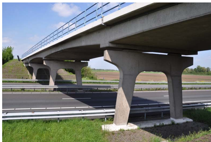
Figure 1. Zijlweg bridge (viaduct) in the highway A59 in the province Brabant, the Netherlands.
