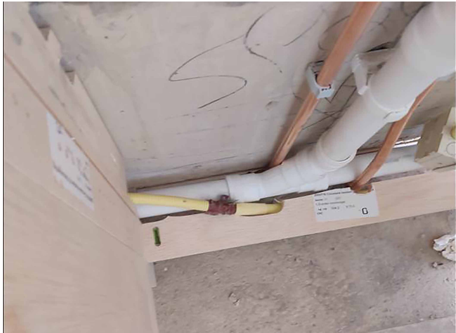
FIG. APP.C.14 Existing plumbing 'colliding' with parts of the CIK demonstrator kitchen
