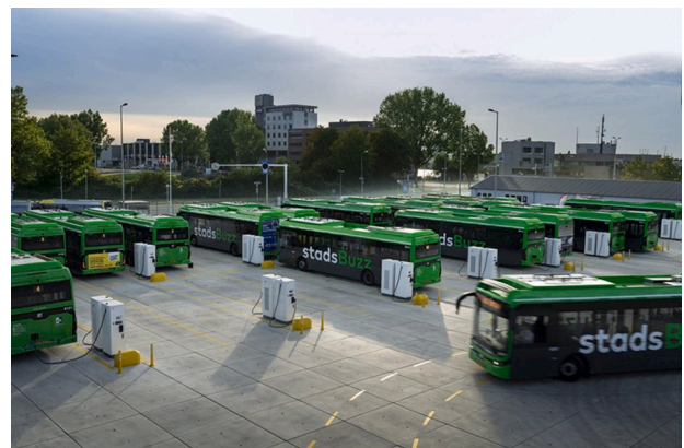
Fig. 6. Depot chargers for heavy vehicles (EVs, C., 2022 ).
