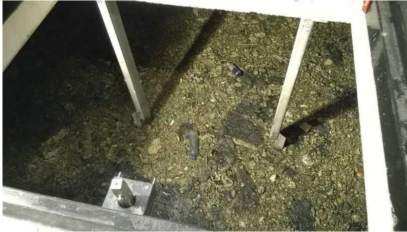
Figure 1 The presence of a closed floating layer of scum and fat in a wastewater pump sump (Rotterdam, 2014)
