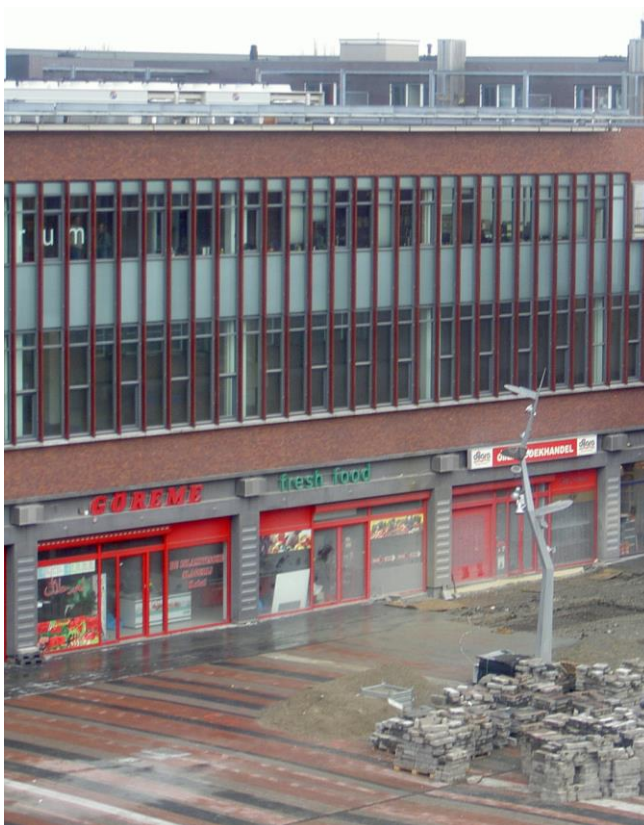
Figure 7.1 Recovery activities at Bos & Lommer Plaza (photo: Dick Hordijk)
