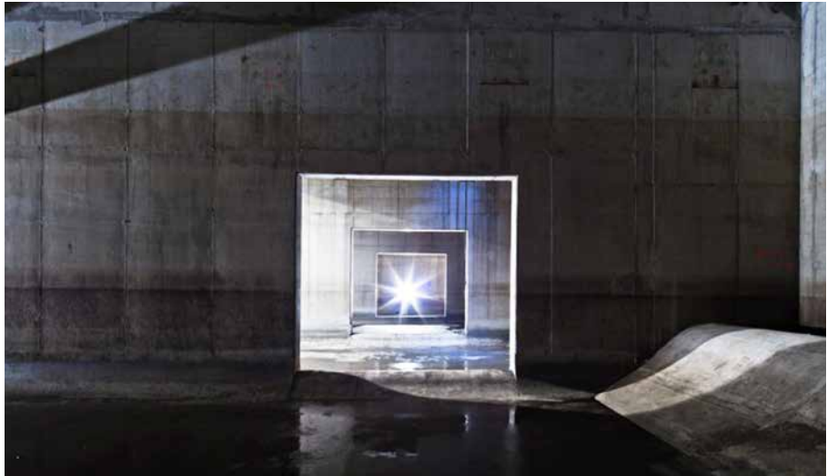
FIGURE 9.27 Water storage for heavy rainfall under parking garage Rotterdam (source: IABR.nl)
