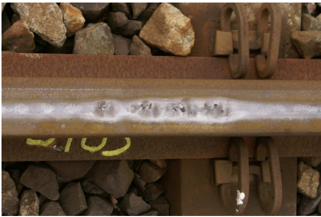
Fig 1: Example of severe squats on a rail
