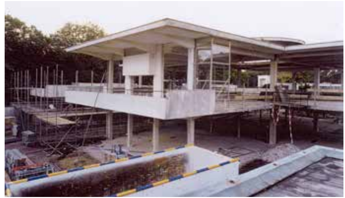
FIG. 2.16 After the removal of all later additions and alterations, this is all that was left of the original substance of the Main Building of Sanatorium 'Zonnestraat'. The upper corner shows the first test for the new glazing / Wessel de Jonge Architects
