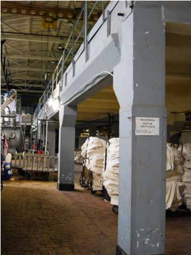
FIG. 3.27 The combined concrete frame and steel trussed structure of a former textile factory, Vishny Volochnik / Marieke Kuipers
