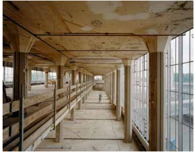
FIG. 3.31 The concrete structure of the Van Nelle Factory, Rotterdam, with 8-sided mushroom columns, inside the curtain wall of glass and steel / courtesy of the Cultural Heritage Agency of the Netherlands
