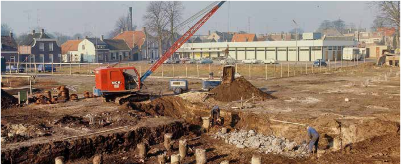
FIG. 3.24 A construction site with old concrete piles exposed, Oosterhout / courtesy of the Cultural Heritage Agency of the Netherlands
