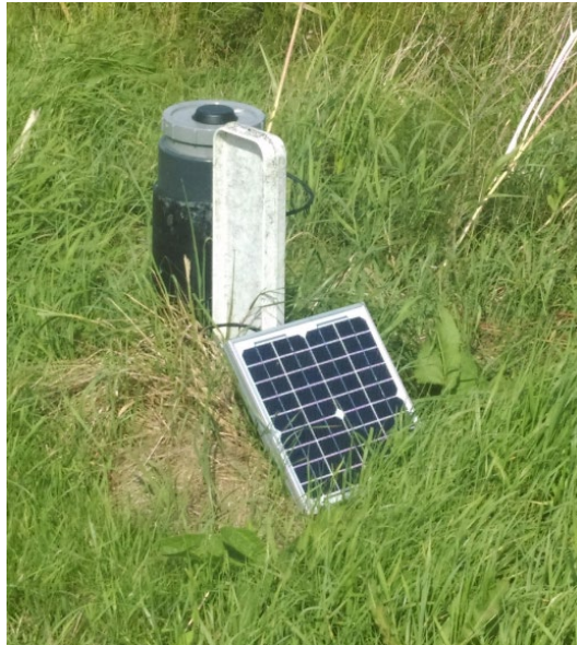
Figure 4-11: Automatic water level measuring station ( https://waterwindow.nl/casus/peilbuisen-moeilijk-af-te-lezen )
