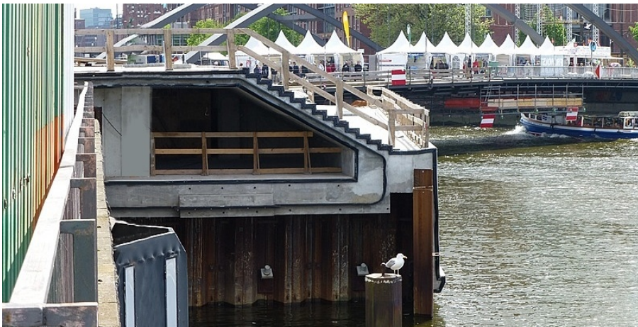
Figure A.21: Hamburg: multifunctional quay wall near the Baumwall under construction, May 2012
