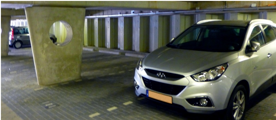
Figure A.11: Zwijndrecht: The parking garage under the Maasboulevard, May 2012. The sheet pile wall behind the car is water-retaining
