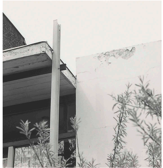
FIG. 1.3 Plasterwork and wood exhibited serious blemishes
