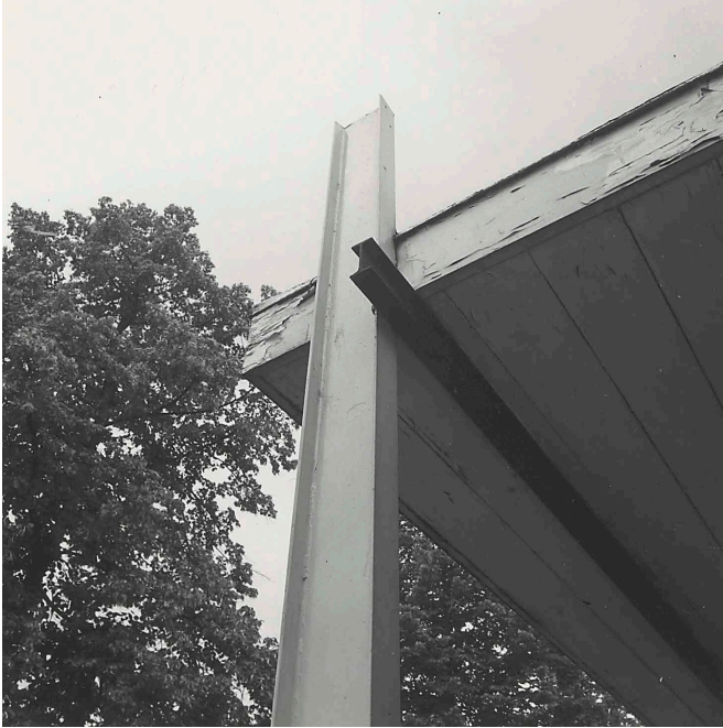
FIG. 1.4 Unconventional constructions made the house vulnerable
