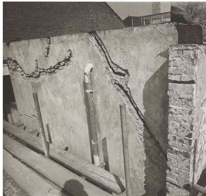
FIG. 1.9 The brickwork displayed deep cracks
