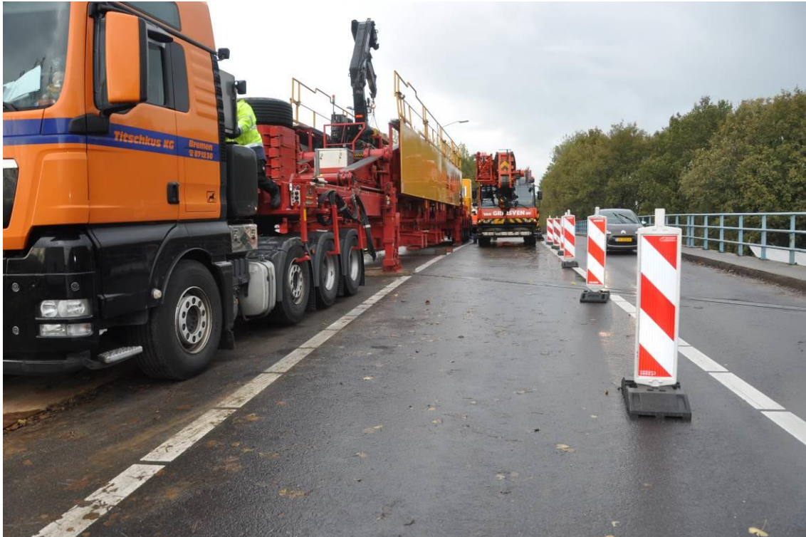
Figure 3. Proof load test on viaduct where one lane of traffic (right side of photograph) remains open for traffic (Fennis et al. 2014, Koekkoek et al. 2015).
