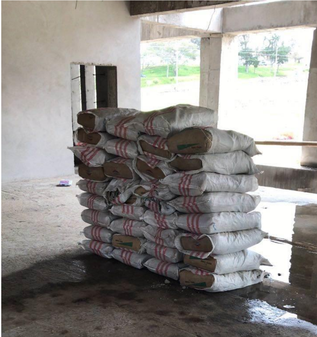
Figure 13. Example of application of dead weight with cement bags. Photograph by S. Camino. Printed with permission.
