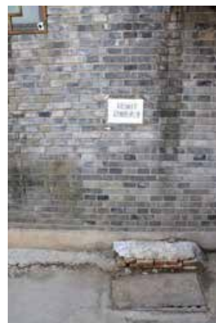
Figure 4. The covered catch basin and the warning sign on the wall (Source: author photo)
