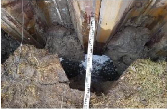
Figure 16. Gapping behind sheet pile wall AZ26
