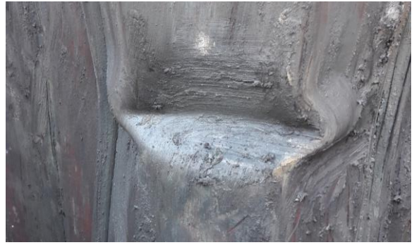
Figure 14. Excavated GU8N-rev with local buckling
