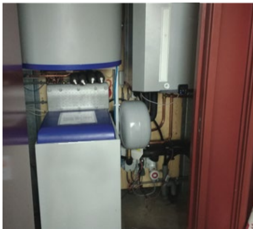
Figure 6 The installation room in a ZE house. It houses the equipment, but is a black box to residents.
