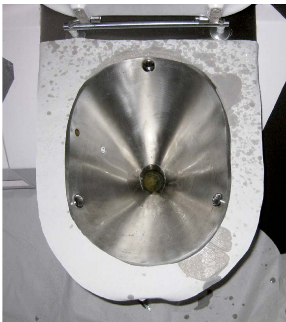
Figure 5.9 Spillage on toilet seat and floor using paper
