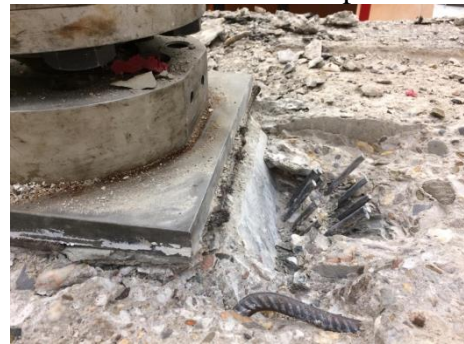
Failure, top view showing anchorage of prestressing tendon
