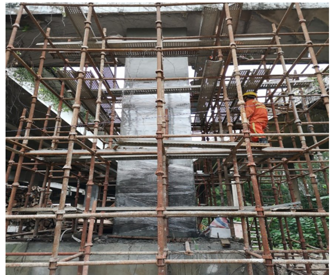
FIGURE 2 Installation of impressed current cathodic protection-structural strengthening (ICCP-SS) system on piers of the Guangzhou-Shenzhen highway
