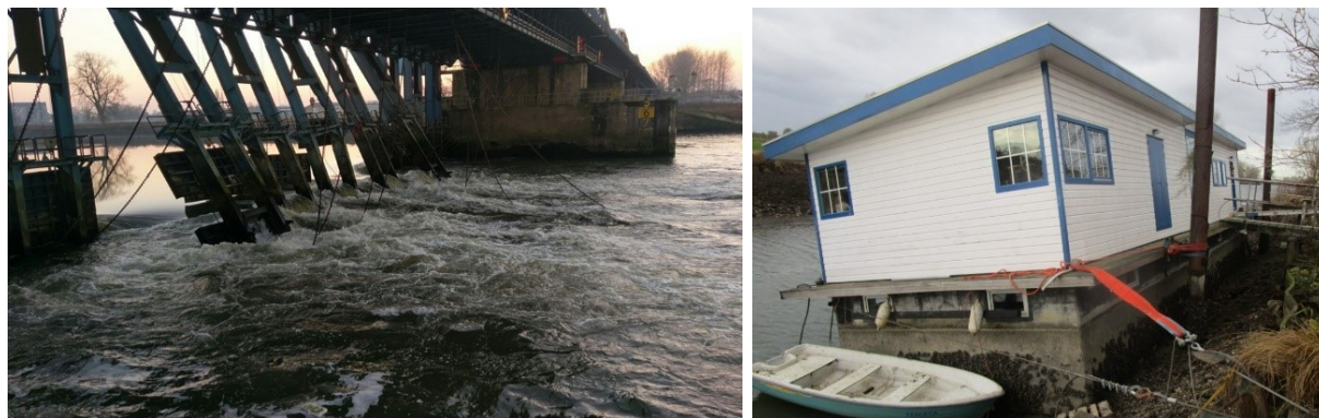
Figure 3.25: Damage to the weir at Grave (left) and the consequences upstream (right) (left: Stuw Grave aanvaring by Nico van Lammeren is licenced under CC0 1.0; right: BootAanBoot.NL , all rights reserved).
