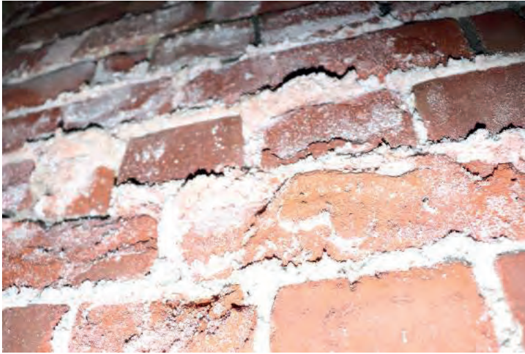
Figure 2: Brick surfaces and salt at the south side of the brick chimney in October 2019
