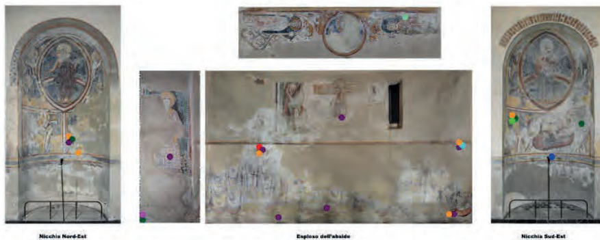
Figure 9: Distribution of salt efflorescence on painted walls. Red dot: epsomite; orange dot: gypsum; blue dot: hydromagnesite; light blue: magnesium carbonate; purple dot: calcite; pink dot: thenardite; green dots: other substances (biological colonization) and polymeric film layer.
