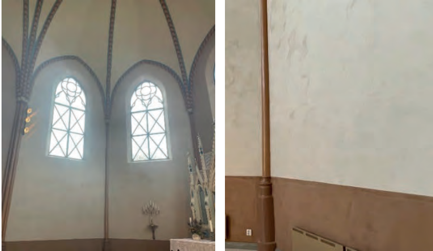
Figure 5: The two walls that have been plastered with hemp-lime in the choir. After two years there are no signs at all of salts on the surface. Only the normal liveliness of the lime wash gives the surface its expression.
