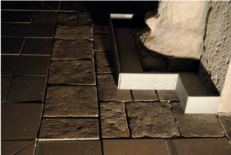
Figure 3: Floor plates with open joints and boxes made of wood to sample the fell off for the monitoring.
