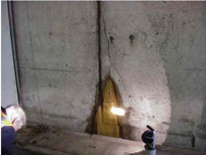
Figure 3. Cracking at segment joint.
